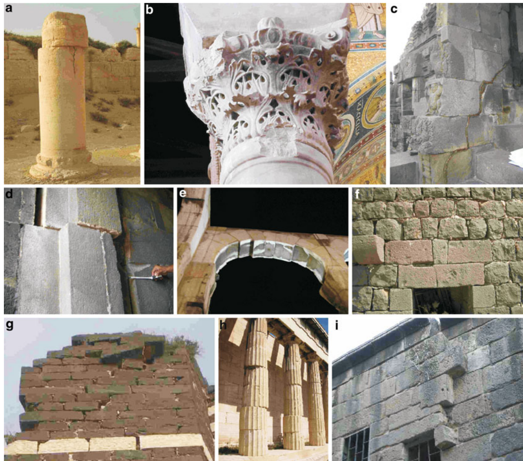
Fig. 1 Typology of earthquake-induced damages in ancient buildings. (a) Cracks/fractures within a block (second century AD Palmyra theater, Syria). Photo Kázmér #4281. (b) Chipped edges of column and capital in the sixth-century Euphrasius cathedral, (Poreč, Croatia), damaged by the 1440 earthquake #0080. (c) Through-cutting fractures (repaired) in the eight- to ninth-century Brahma temple of the Prambanan complex, Yogyakarta, Indonesia, caused by the 2006 earthquake #6488. (d) Horizontal shift of large ashlars; vertical joints opened up between them. Shiva temple, Prambanan complex, Yogyakarta, Indonesia. Tape measure extended 20 cm #6498. (e) Dropped ashlars in a Roman arch (Damascus, Syria) #2017. (f) Broken lintels in twelfth-century al-Marqab citadel, coastal Syria #4663. (g) Clockwise-rotated blocks in twelfth-century al-Marqab citadel, coastal Syria #5168. (h) Displaced drums of masonry columns of the fifth-century BC Hephaisteion temple, Athens, Greece #1132. (i) Extruded portion of house wall. Bosra, Syria #4183
