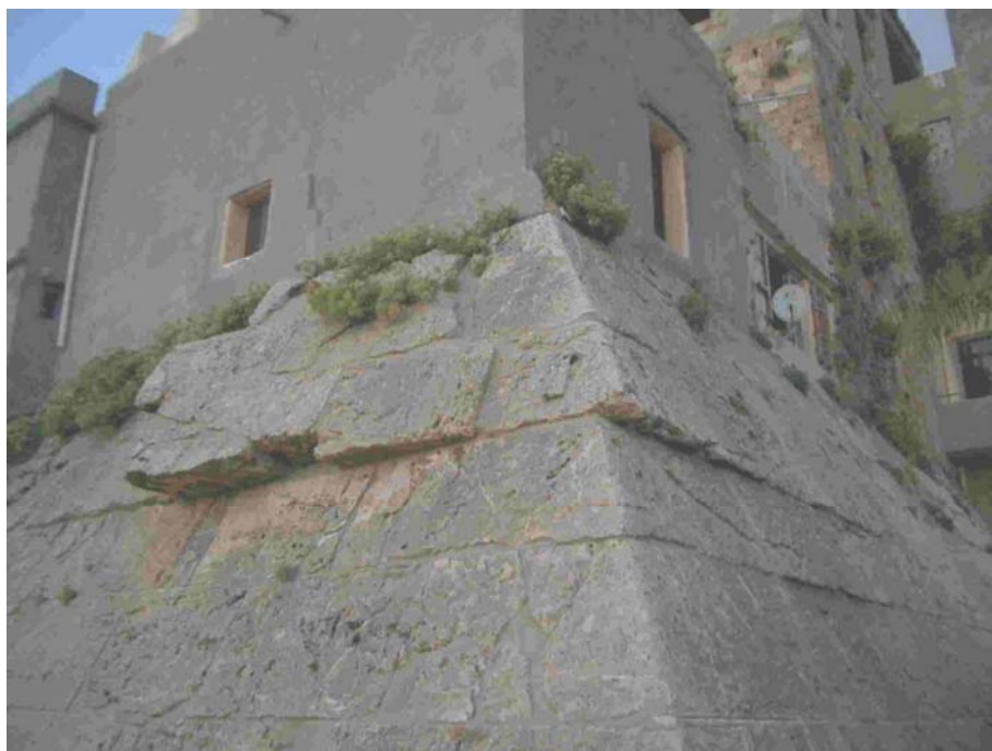
Fig. 6.55. Rotated blocks within the sea wall of the crusader castle, Tartous, coastal Syria ( 39^{\circ} 53' N , 35^{\circ} 52' E ). The fortress, built in the 12th century by the knights of the Temple, suffered the greatest damage probably during the 1202 AD earthquake. Blocks are ca. 70 cm high. The counterclockwise rotation of four blocks together (left block towards the viewer) was caused by E-W strong seismic motion. There is a right-lateral strike-slip fault on the northern side of the leftmost blocks. Vertical component of seismic waves allowed the blocks to rotate when the overburden was momentarily relieved, and seismic loading overcame friction. Photo #4682.
