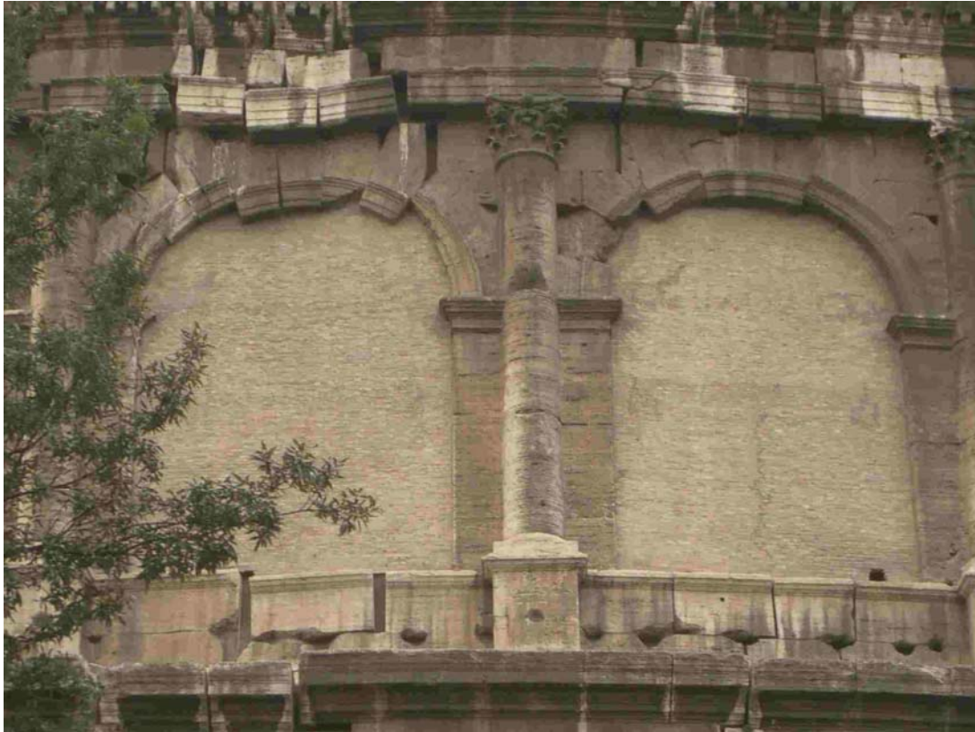
Fig. 6.54. Dropped keystones and adjacent blocks in the arches of the Colosseum, caused by earthquake shaking. The feature is a miniature analogue of rifting: extension produced open fissures, normal faulting, subsidence and tilting of blocks.
