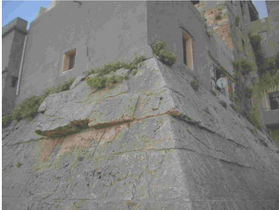
Fig. 6.55. Rotated blocks within the sea wall of the crusader castle, Tartous, coastal Syria (39° 53' N, 35° 52' E). The fortress, built in the 12th century by the knights of the Temple, suffered the greatest damage probably during the 1202 AD earthquake. Blocks are ca. 70 cm high. The counterclockwise rotation of four blocks together (left block towards the viewer) was caused by E-W strong seismic motion. There is a right-lateral strike-slip fault on the northern side of the leftmost blocks. Vertical component of seismic waves allowed the blocks to rotate when the overburden was momentarily relieved, and seismic loading overcame friction. Photo #4682.
