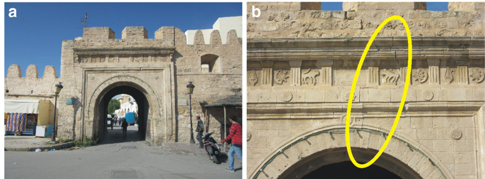
Fig. 8 Slightly damaged arch of the southern gate to the medina , Monastir. a Monastir, medina , southern gate. #6193. b Left part of gate subsided. Displacement extends up to the ledge, going around all masonry blocks (circle). #6194. I = VII. 35^{\circ} 46' 22'' N, 10^{\circ} 49' 50'' E
