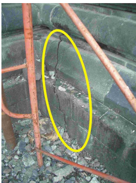
Fig. 6: Brahma temple: a NW-SE left-lateral fault cross-cutting the temple diagonally. A reinforced concrete wall surrounds the level below this floor. There was 4 mm left-lateral displacement.
