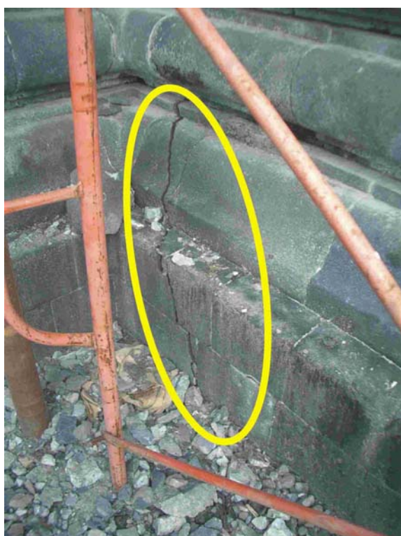
Fig. 6: Brahma temple: a NW-SE left-lateral fault cross-cutting the temple diagonally. A reinforced concrete wall surrounds the level below this floor. There was 4 mm left-lateral displacement.
