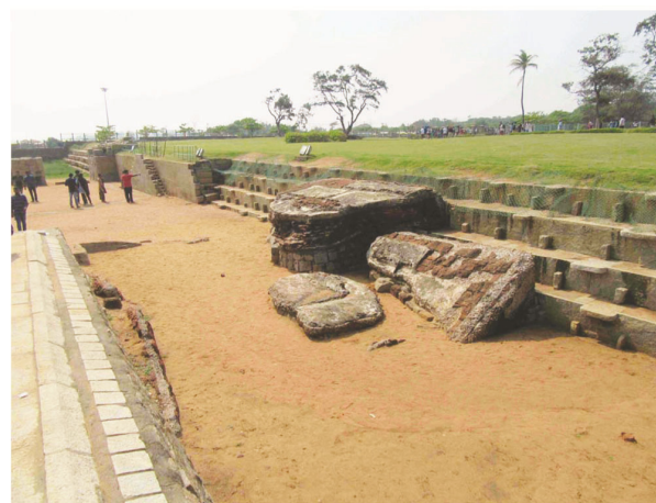
Figure 6. Collapsed walls and floor level of a brick building in the Shore Temple complex at Mahabalipuram. Tilted walls are evidence of liquefaction. Note vertically tilted wall on the left of the sandy floor. Persons in the background for scale. ADB Photo #2166.
