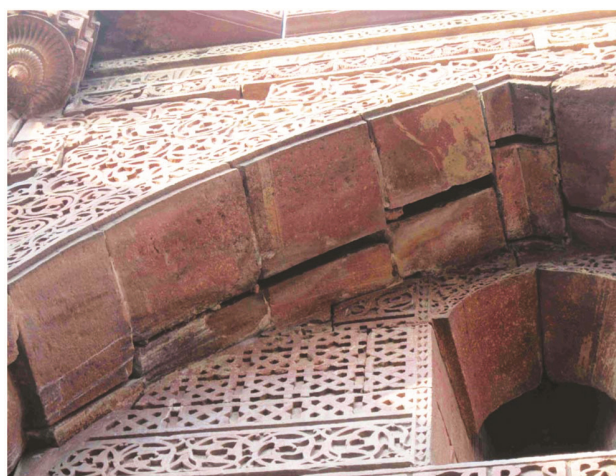
Figure 3. Inner facade of the northern gate in the Tomb of Iltutmish, Qutub Minar complex in Delhi. Out-of-plane shift of arch masonry blocks separated by more than 5 cm wide gap nearby the top of the entrance arch. Photo #1941.
